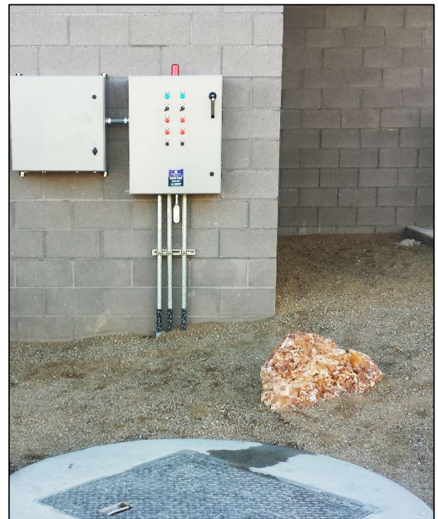
This control panel is within view of the wet well and installed at a comfortable working height; about 3'-4' above finish grade.
