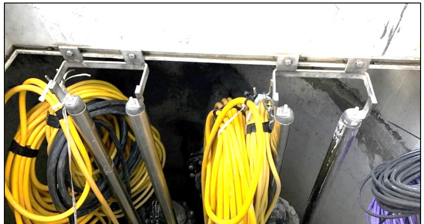
After cable ends have been pulled to the control panel, excess cable can be coiled and suspended in the wet well on the Jensen-provided hooks.
