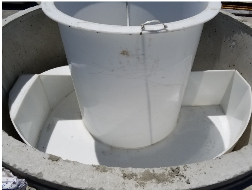
Figure 6. View of Inlet Forebay of “Inline” JDS Unit
